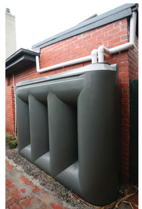
3,000 litre slim line – approx $2,000 inc professionally installed.
